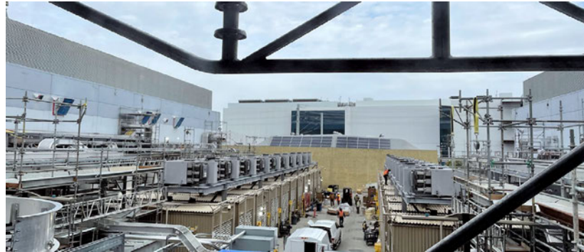
This west coast data center in Santa Clara, California, installed 25 active diesel particulate filters to the existing MTU S4000 engines to comply with regulatory standards, significantly reducing emissions and maintenance workloads.
