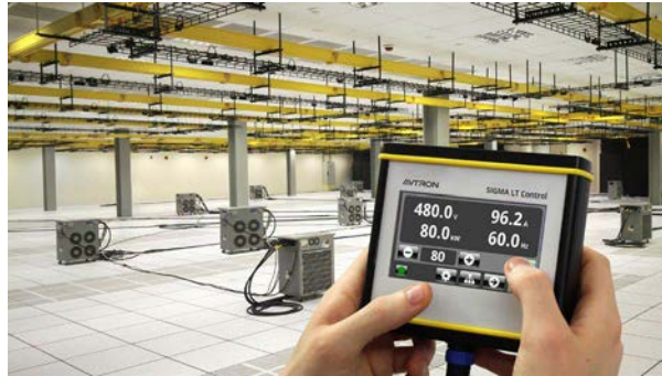
Figure 3 – A sample of load bank test in data center.
